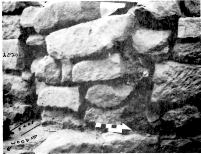
Fig. 10 - 2E20K: View of north side of well entrance showing break in the construction plus stone slot. 6" scale, Facing North. (2E-136-M)
